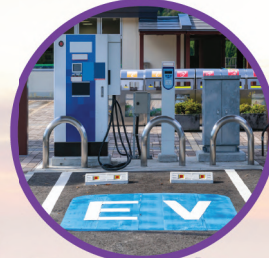
EV Charging Station
